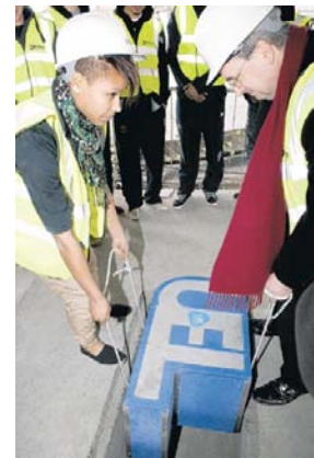
Figure 6: UEL Vice-Chancellor placing a time capsule in the foundations of the SportsDock
